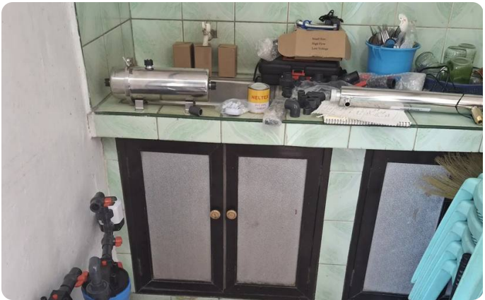
The finished system
