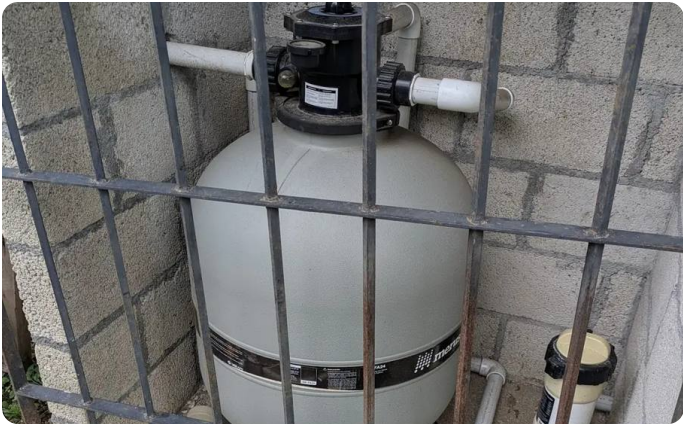
A pressure filter tank in town
