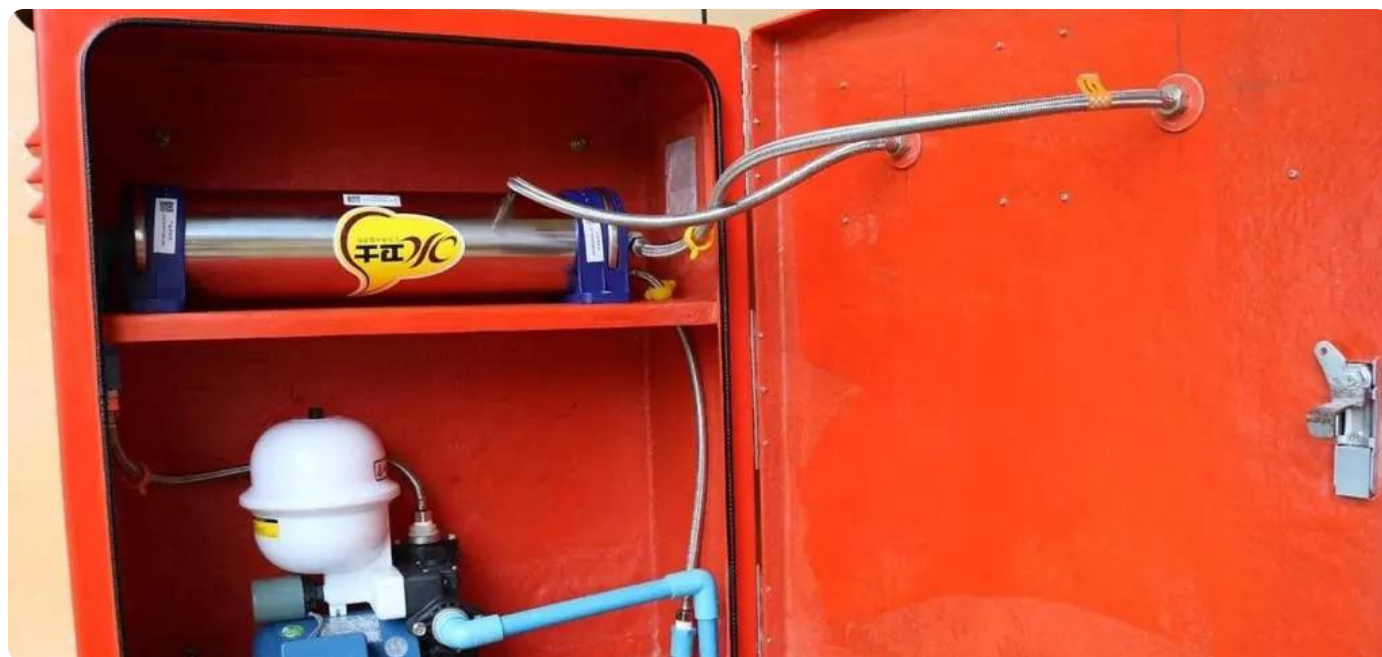
Inside a unit: pump and membrane. Photo: ISZA
