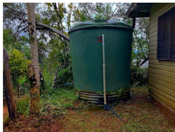
A "Tuffa" storage tank installed beside a building downstream
