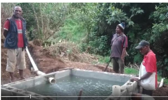
The concrete catchment tank holds and settles incoming creek water
